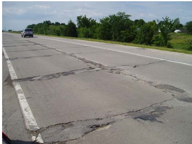
Figure 5. Condition of existing concrete pavement.
