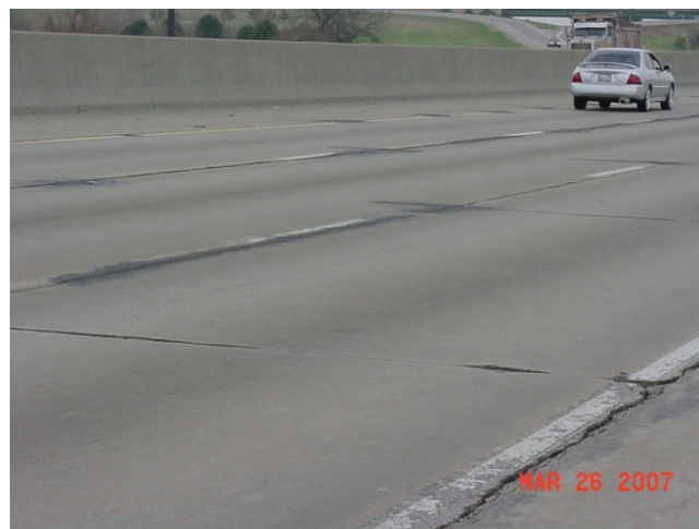
Figure 3. Condition of existing concrete pavement.
