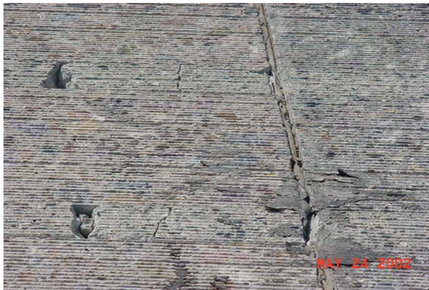
Figure 13. Failure of dowel bar patching material (23).
