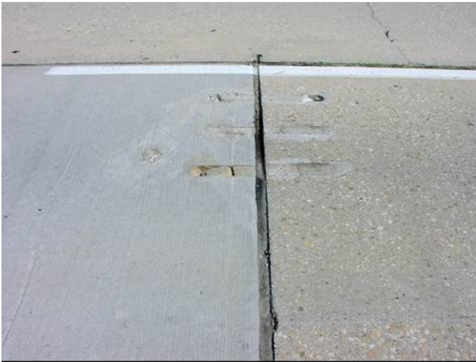
Figure 5. Missing silicone joint sealer.
