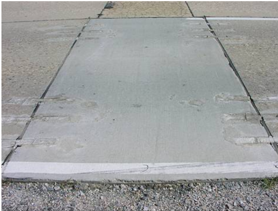
Figure 1. Discontinuous joint at dowel retrofit.
