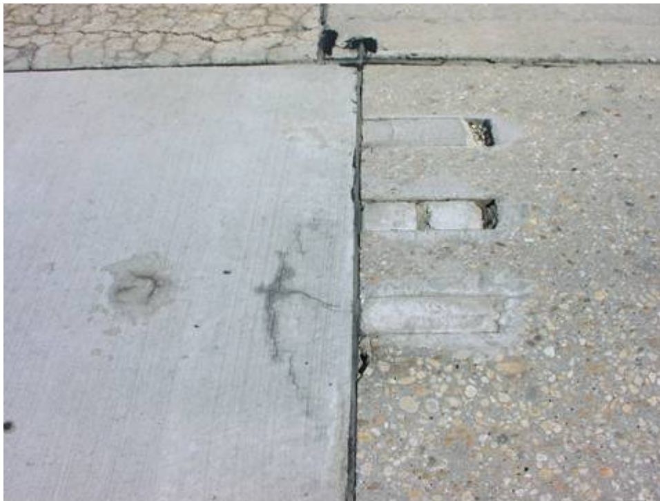
Figure 2. Cracks propagating into patch cast with dowel.
