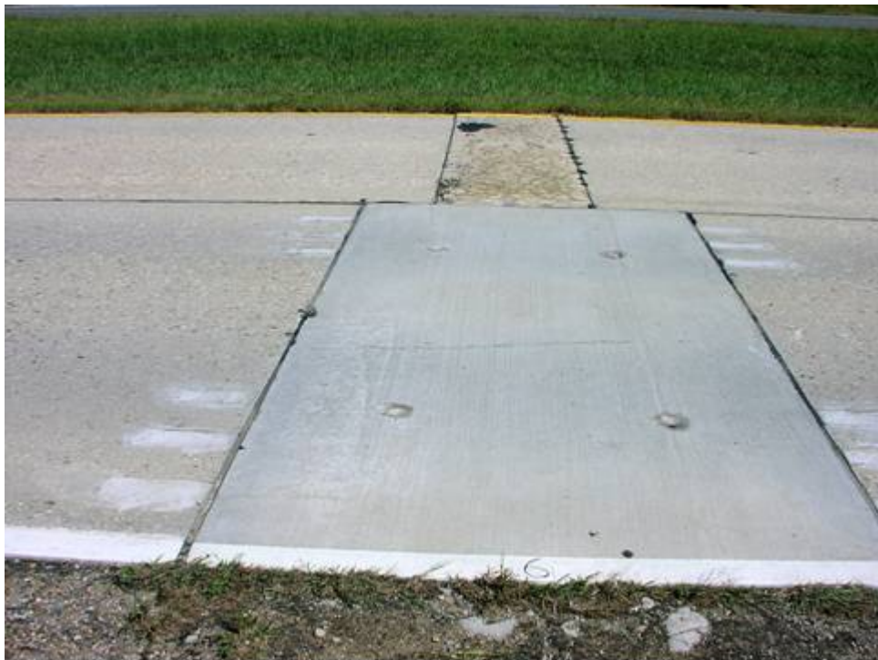
Figure 4. Crack propagating between wheelpaths in patch with cast-in dowel.
