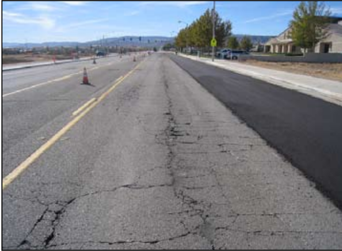
Condition of 60th Street West. Left side shows condition before CIR. Right side shows CIR surface at 3% emulsion content.
