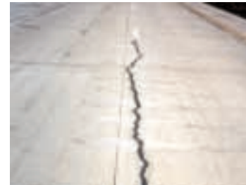
Stitched longitudinal joint and crack.
