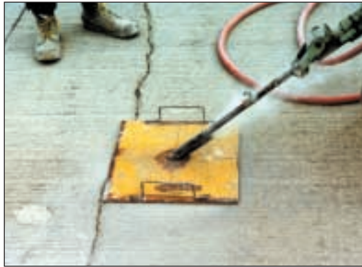
2. Simple drill rig that controls the starting location of drilling to ensure that hole intersects crack at about mid-depth.
