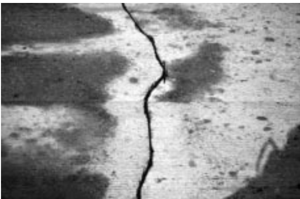
Figure 7.1. A freshly sawed crack.
