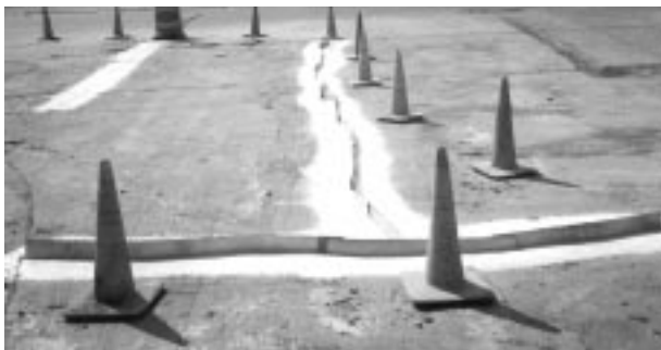
Figure 13.4. Completed partial-depth repairs – note joint re-former as well as heavy coat of curing compound.
