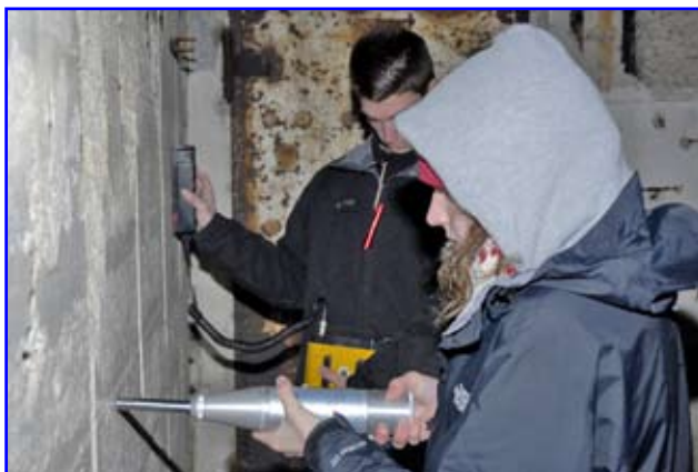
Inside the observation post, Courtney Sheehan tests relative concrete strength with a Schmidt (rebound) hammer while Chad Golden uses a cover meter to determine location, size, and cover of embedded reinforcing.
