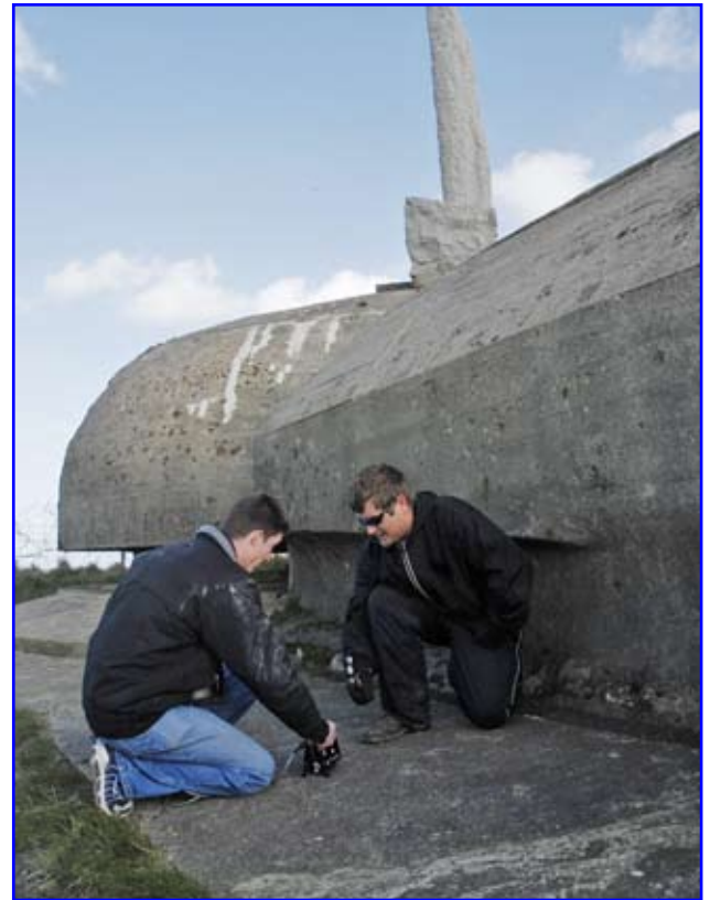
Chad Golden (left) and Andrew Billingsley use Olson Engineering's concrete thickness gauge to determine the thickness of the slab at the exterior of the observation post. The Monument to the Rangers sits on top of the structure.
