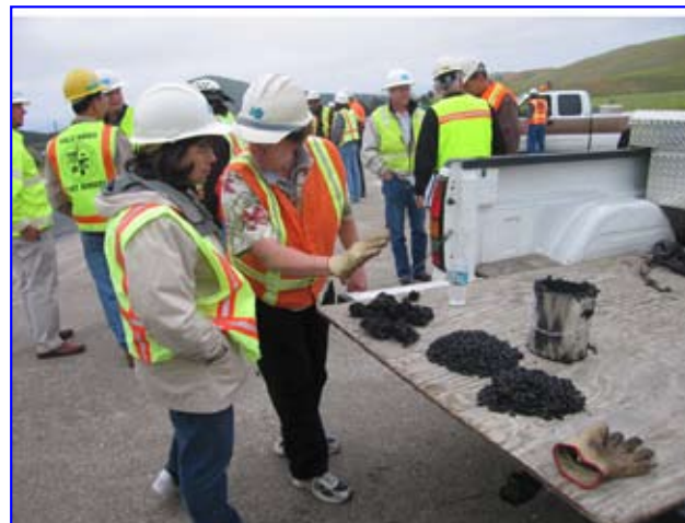
Morro Bay warm mix demonstration project participants discuss the workability of the warm mix obtained from behind the paver.
