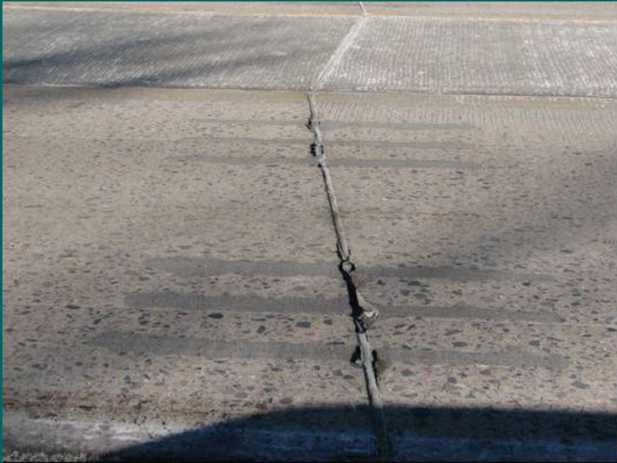
Backfill mortar distress near joint
