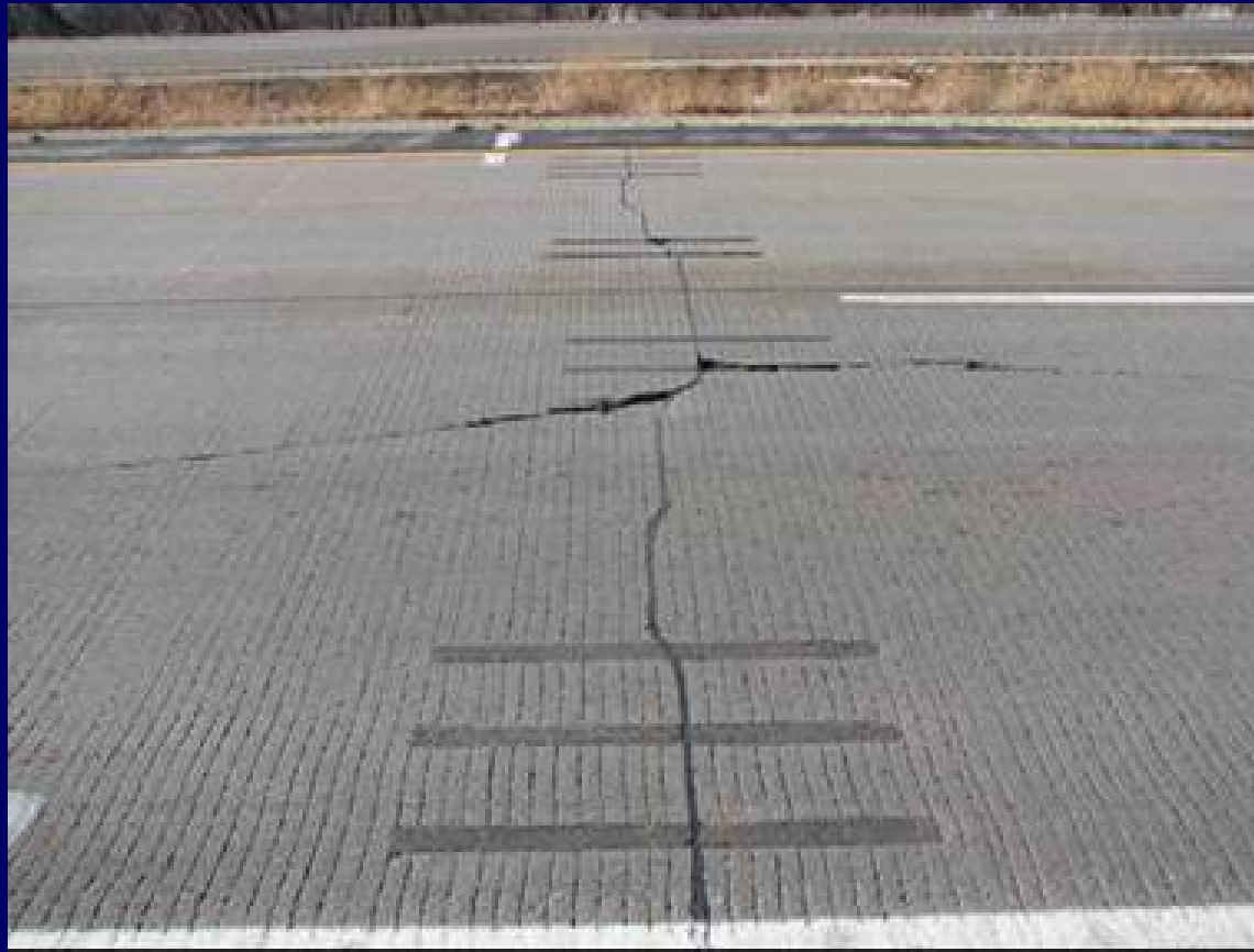
Longitudinal panel crack
