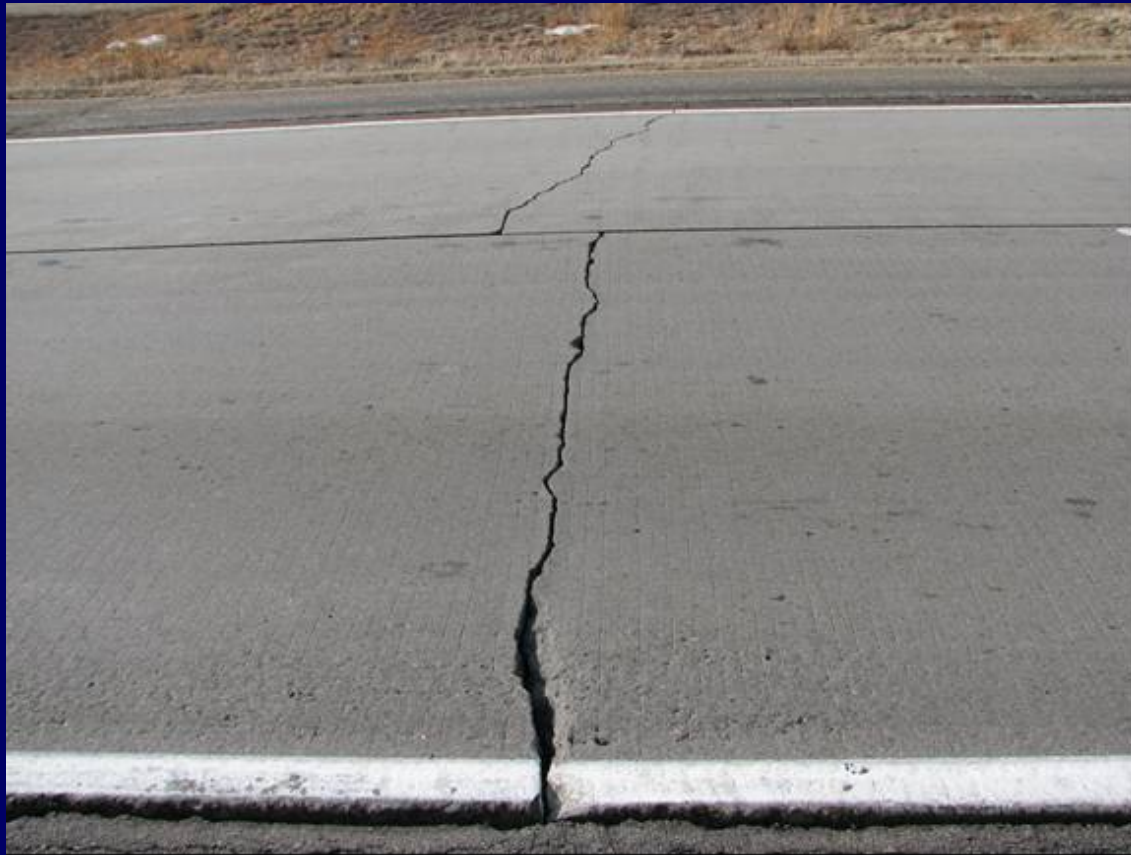
Faulted mid-panel crack
