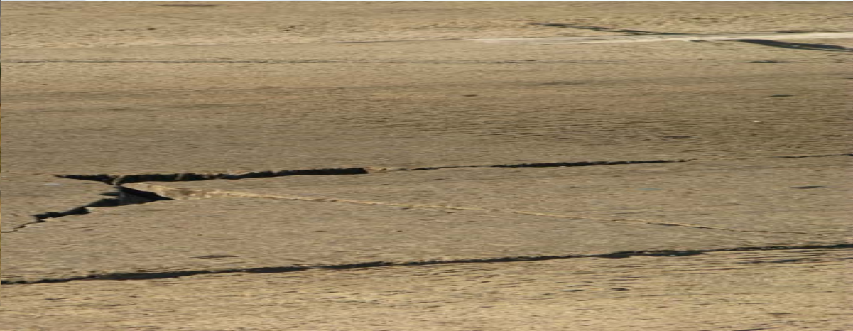
Damaged concrete pavement on freeway lanes
