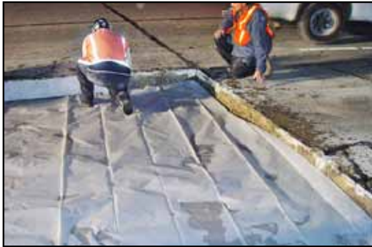
Figure 1. Preparing for pouring of replacement slab. Plastic sheet is a bond breaker.
