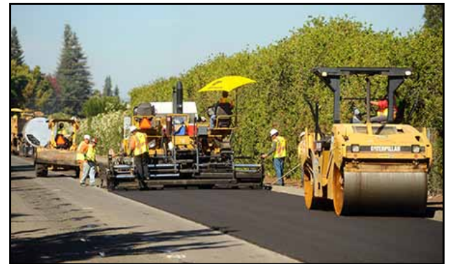
The double steel drum compactor
