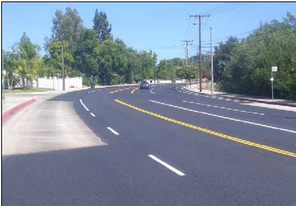
Completed fog seal on Cameron Avenue at Whitebirch Drive in Los Angeles County, California
