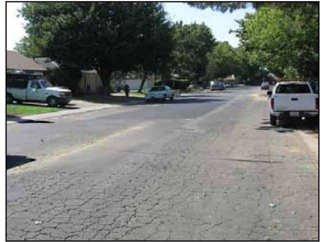
Figure 1. Original pavement condition (Sacramento County, California) prior to interlayer and chips seal application
