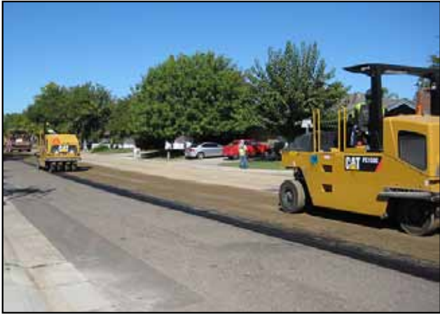
Figure 2. Rolling of interlayer with pneumatic rollers after optional sand application (Sacramento County, California)
