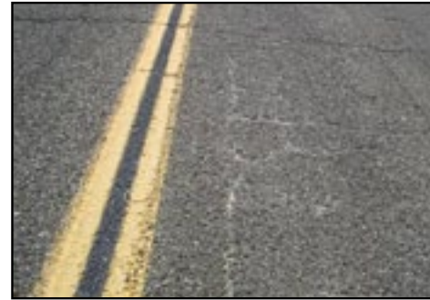
Figure 2. Alligator, longitudinal, and transverse cracking and raveling.
