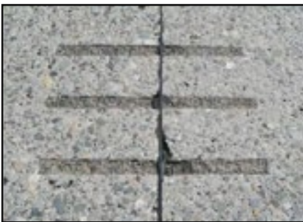
(c) Backfill material spalling
