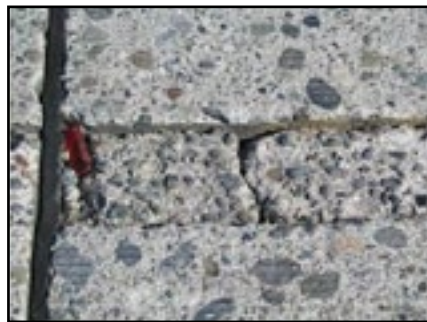
(b) Backfill material cracking
