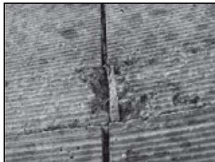
(f) Foam core board misalignment
