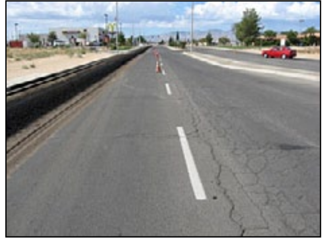
Figure 1. Distresses noted on the project
