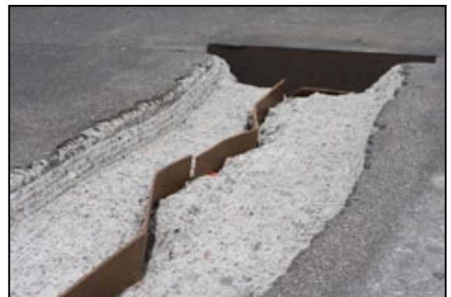
Fig. 3. PDR with joint reformer placed in crack.
