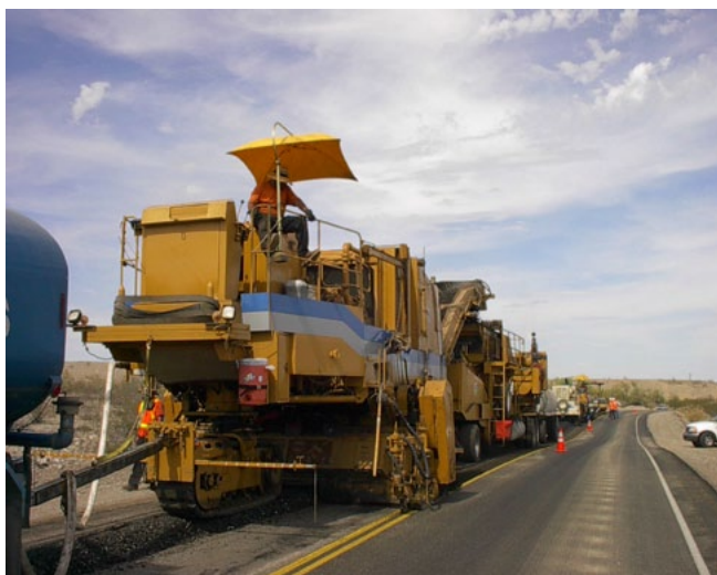
CIR Equipment Train on SR 62. Adjacent Lane Already Recycled with Sand Blotter
