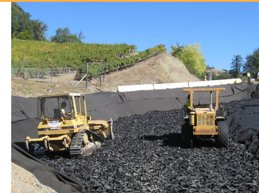
TDA provides long term and cost effective repairs for road failure projects.
