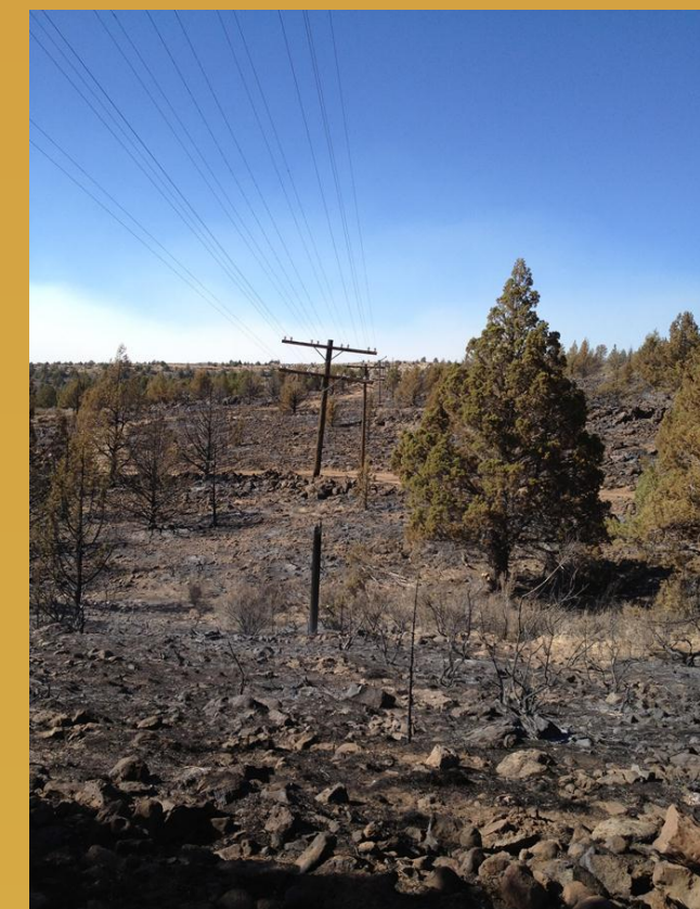
Photograph of damage to historic telephone line by Rush Fire.
